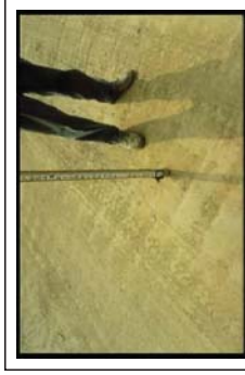
Fig. 3. Construction site with significant compaction of the deep basal till subsoil extends 24 inches below this exposed cut-and-fill work surface.
